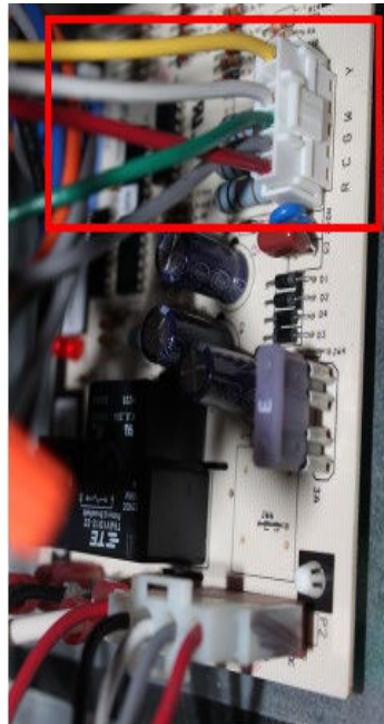
Figure 5: HVAC Equipment Control Board Connection Plug Field connections wire nut to wires (not shown)
